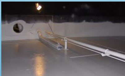
Interior crude oil storage tank
