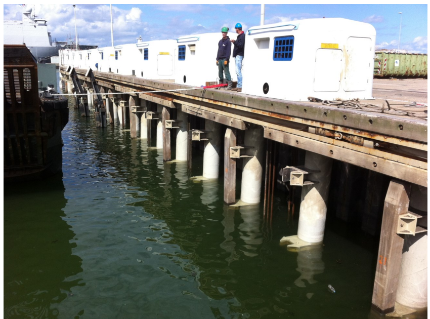
View on the coated tubular piles
