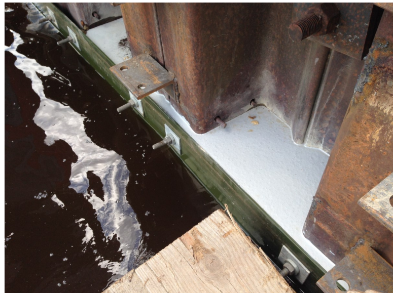
Rehabilitation of severely corroded sheet pile wall with steel plates coated with Humidur
