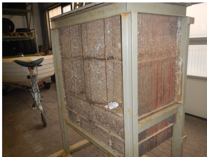
Fouling on the box cooler before treatment
