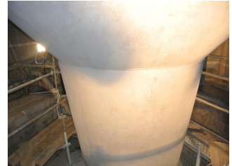
Submerged Kaplan turbine
